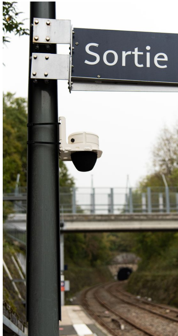
Figure 15: Example of a pod installed on a mast
