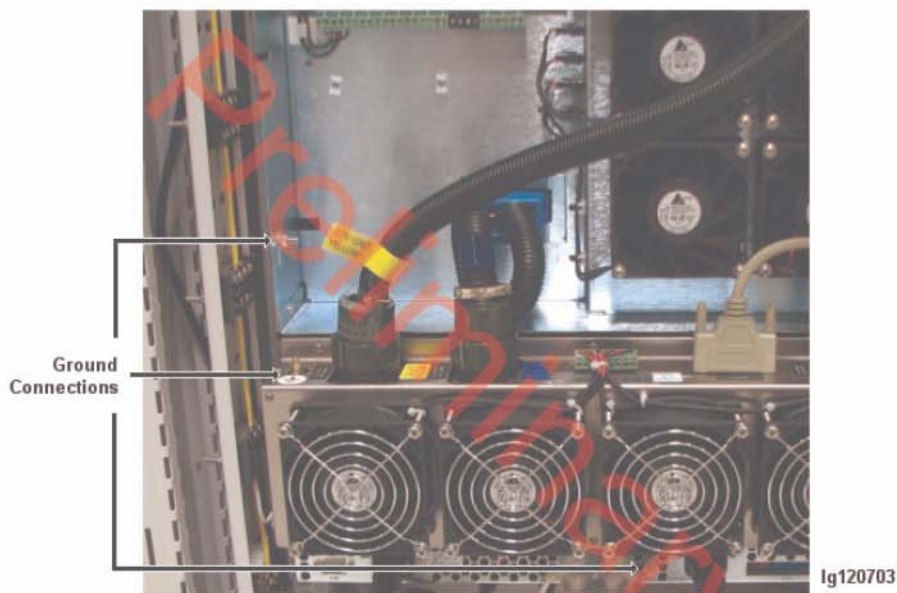
Figure 2-11: Micro Subrack, Power Supply, and Rectifier Ground Lugs
