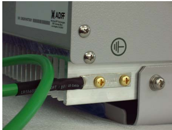
Figure 10 – Ground Cable Connection
