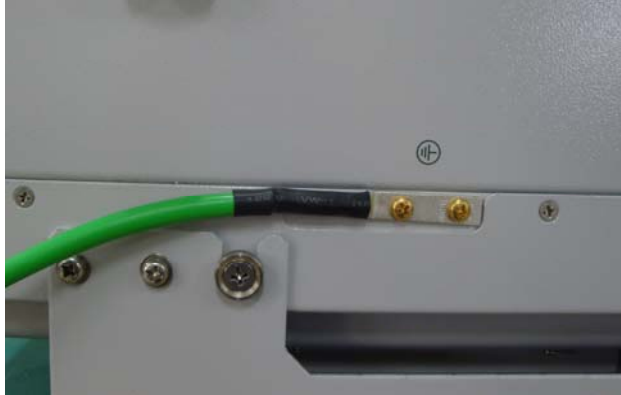
Figure 14: Ground Cable Connection
