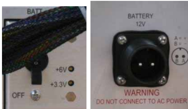
Figure 4: Battery Switch & Battery Port
