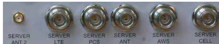
Figure 8: Server Combiner RF port
