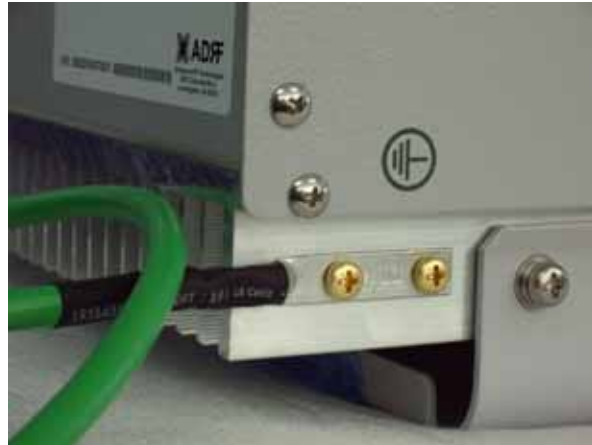
Figure 5: Ground Cable Connection
