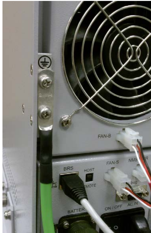
Figure 8: Ground Cable Connection
