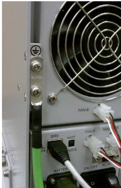
Figure 8: Ground Cable Connection
