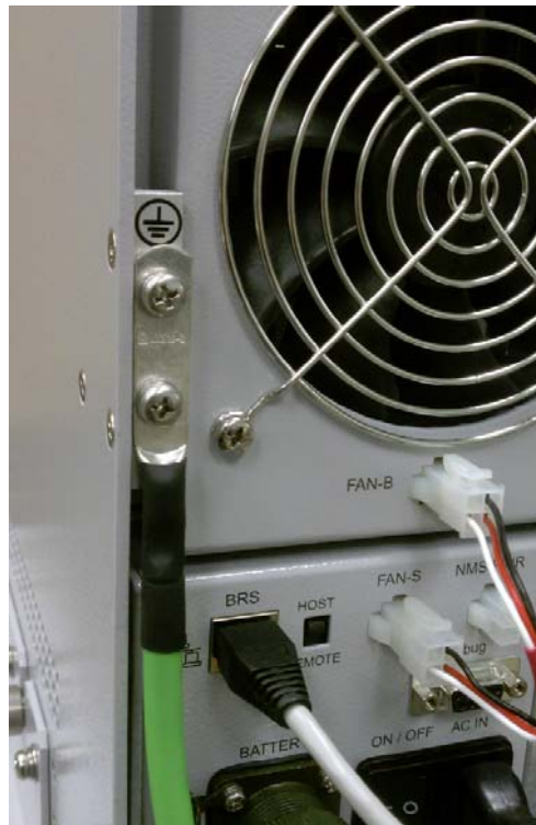
Figure 8: Ground Cable Connection
