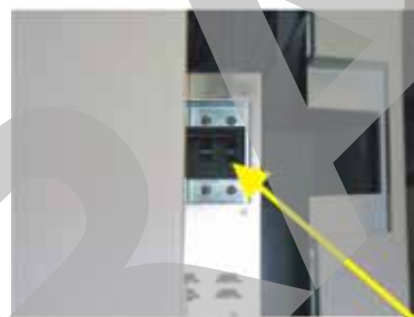
Main Circuit Breaker
