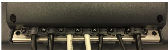
Fig. 6.9: Cable cover closed and screwed together
