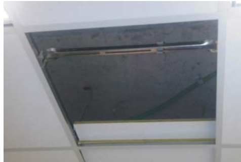
Figure 12: Exciter Mounting Clip positioned on a grid of a false ceiling
