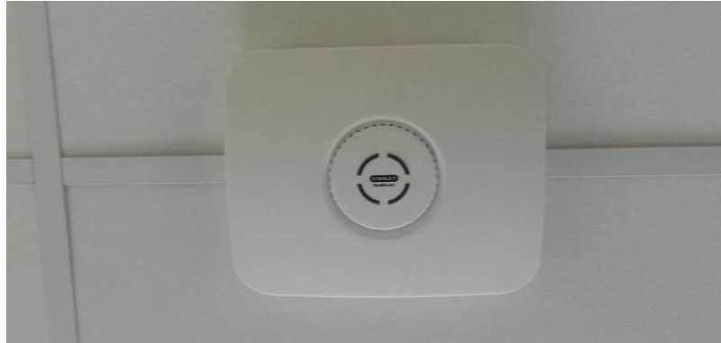
Figure 9: Controller mounted on a Floating Ceilings
