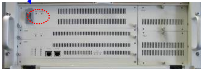
Figure 4-14 RCPB Panel Photo
