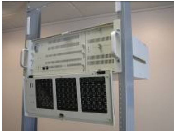
Figure 3-3 – Typical OneRAN Pilot Station Rack Mounted
