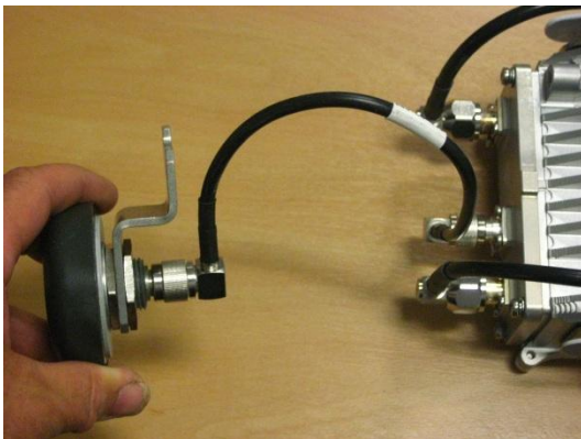
Figure 26 –GPS antenna cable connected
