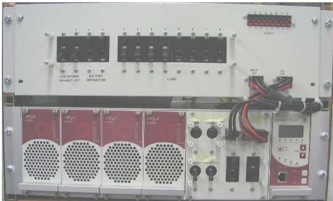
Figure 7-4: BPS Main Rack front view
