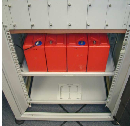
Figure 7-6: Cabinet battery area
