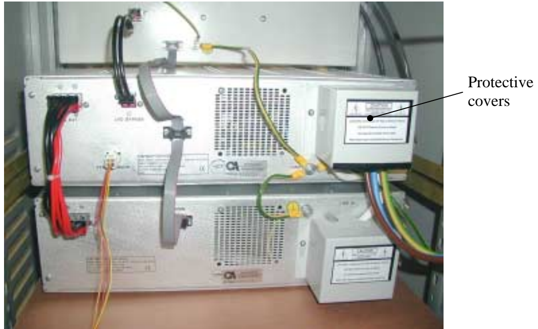
Figure 7-7: Rear BSPS cable connections
