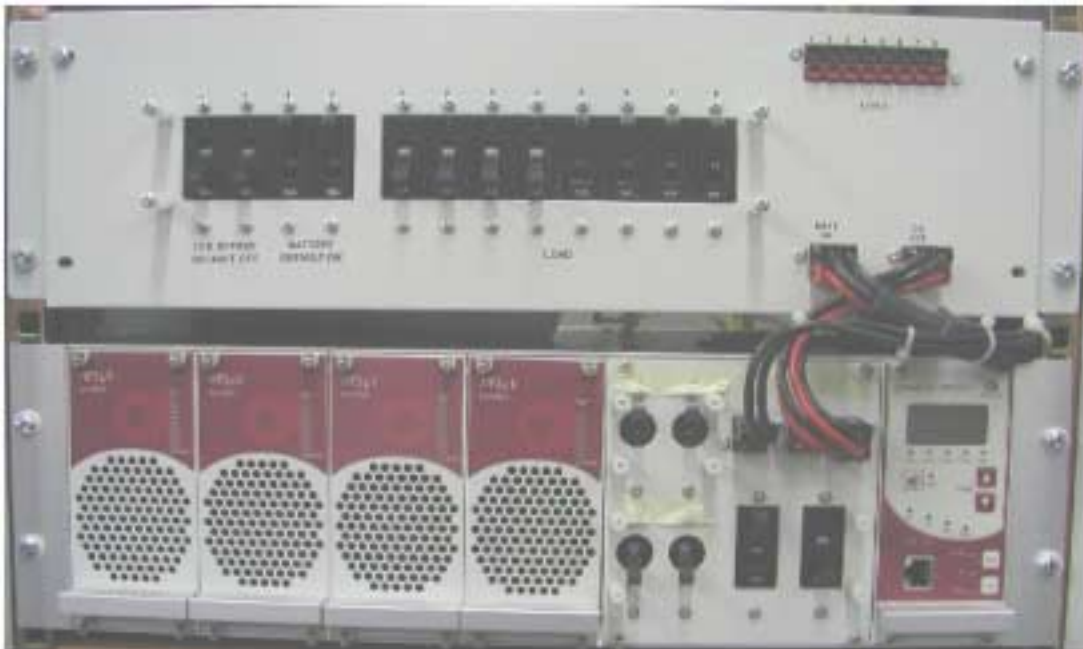
Figure 7-6: BPS Main Rack front view
