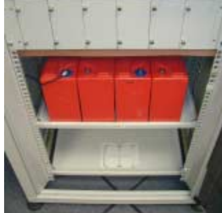
Figure 7-4: Cabinet battery area
