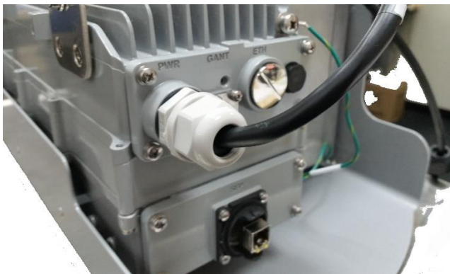
Figure 31: Power cable attached to AirHarmony-1000D
