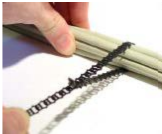
Figure 62 – Secure fiber-optic cable, pull tie
