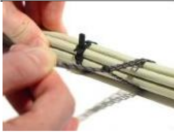
Figure 54 – Secure fiber-optic cable, use excess tie
