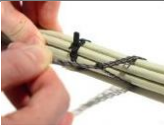
Figure 37 – Secure fiber-optic cable, use excess tie
