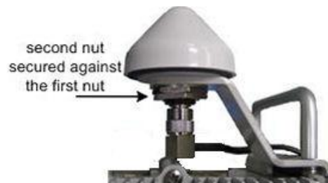
Figure 16 - GPS antenna assembled on bracket
