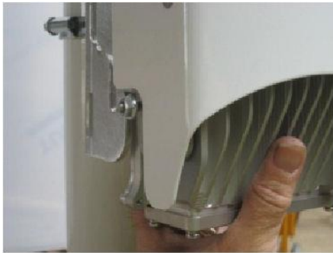
Figure 25 - Gently lift the unit until the bottom studs fit into the bottom slots
