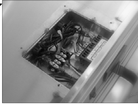
CONTROLLER LOCATION AND MAIN POWER SWITCH (COVER REMOVED)
