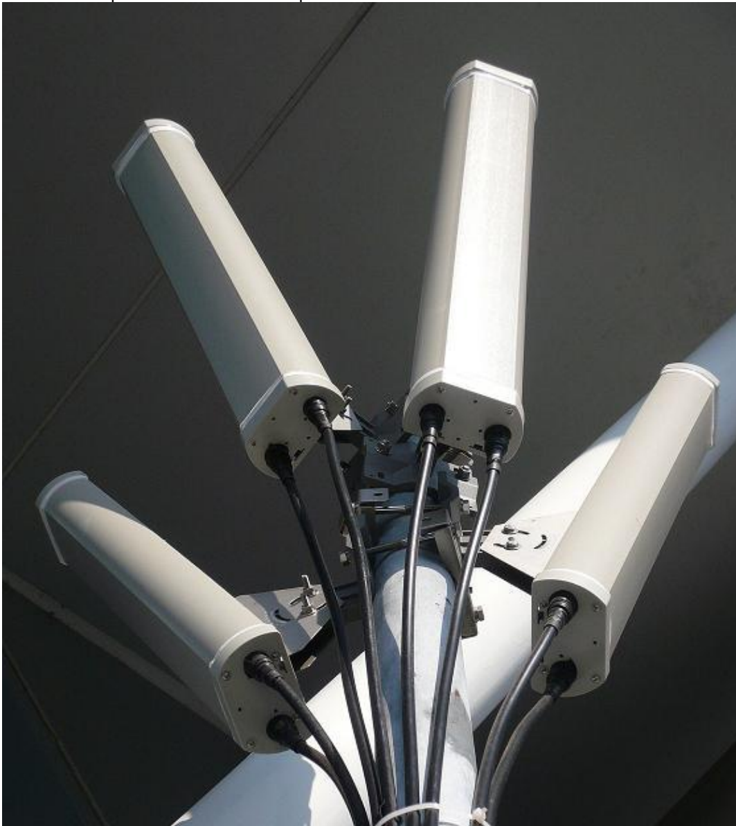
Figure19. RF cable connection from panel antenna
