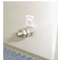
Fig. 14: ground terminal on the rear
