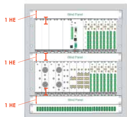
Fig. 4.1.11: intra-subrack distance must be at least 1HE to allow air circulation. 1-HE inter-subrack distances can be properly filled through blind panels
