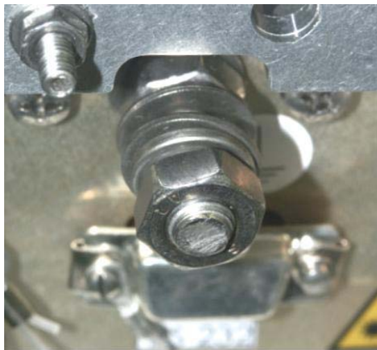
figure 3-7 Grounding bolt with loosened hex nut
