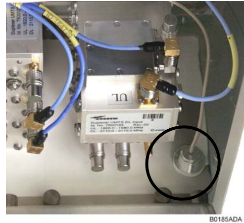
figure 5-14 Cable from modem to external modem antenna port; Node M
