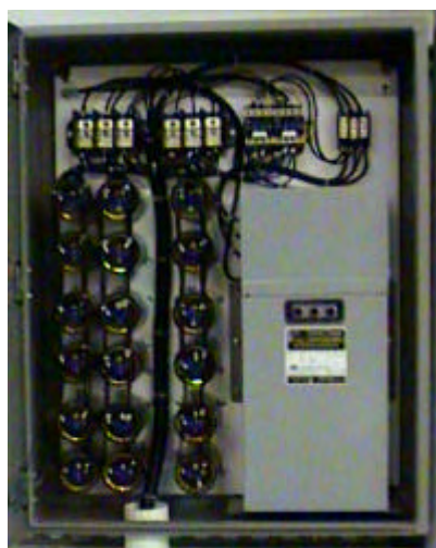
Figure 12.1-2 Dynamic brake capacitor enclosure and power factor correction
