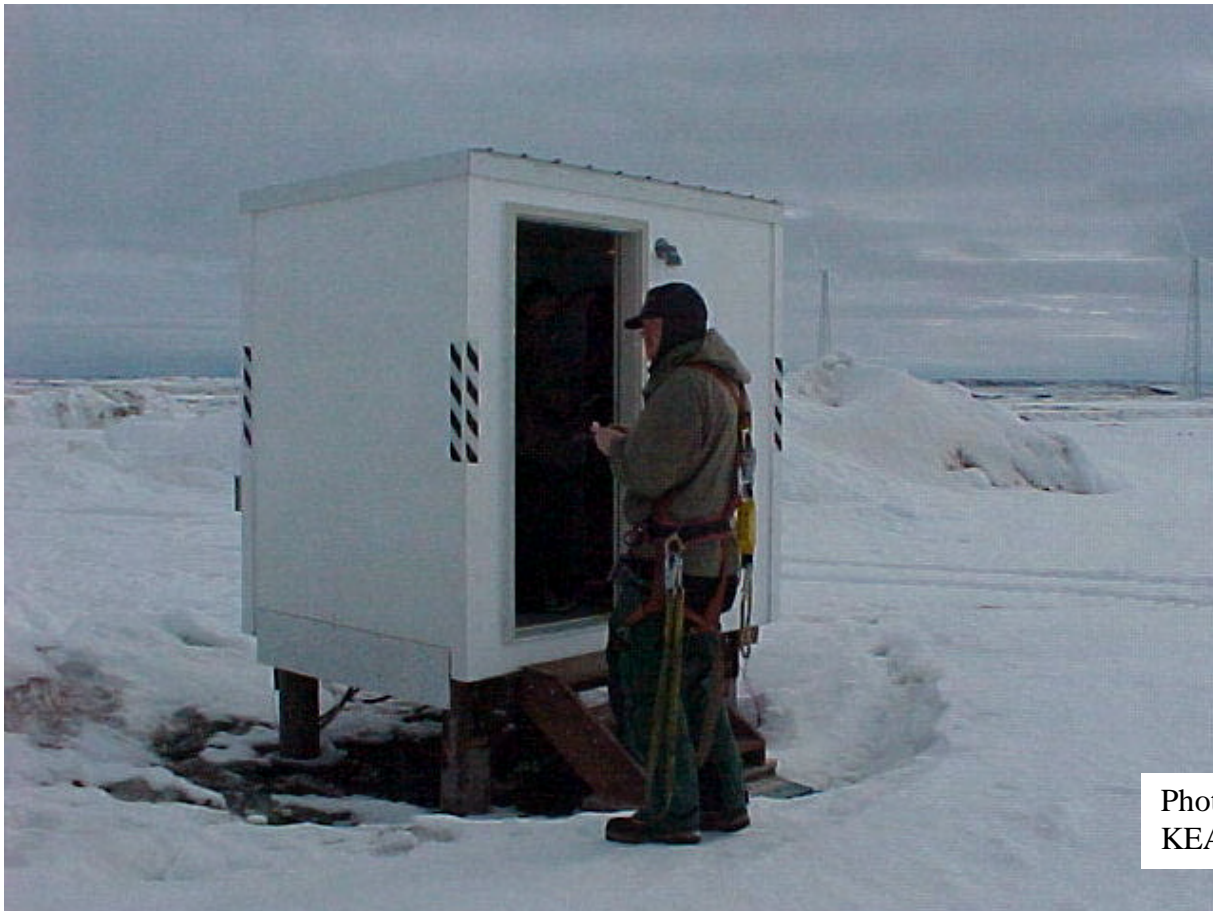
Figure 7-5 Control box at Kotzebue Electric Association
