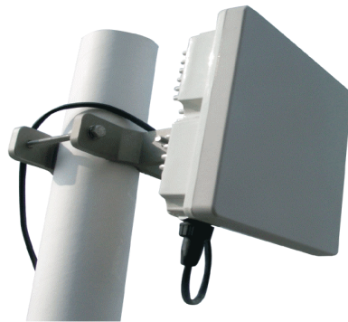
Figure 2-6 Installed PacketMax 100-ODU
