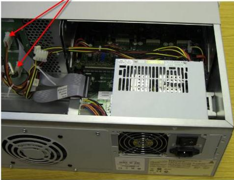
Power unit cables connected to the BCM's Main Chassis
