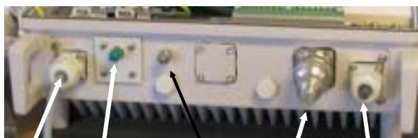
Power Fiber connector Ground Server antenna External alarms
