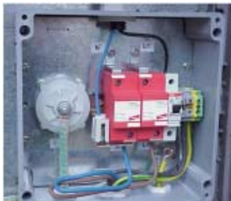
Protective device installed in connection with the power supply
