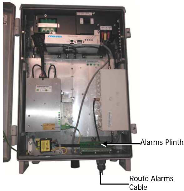
Figure 2-29. Example of Repeater Showing the Location of the Alarms Plinth
