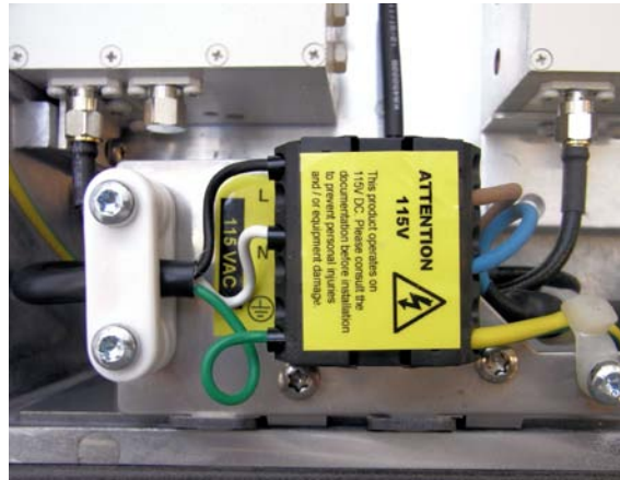
Figure 2-25. 115VAC Power Connections
