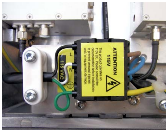
Figure 3-34: 115VAC Power Connections
