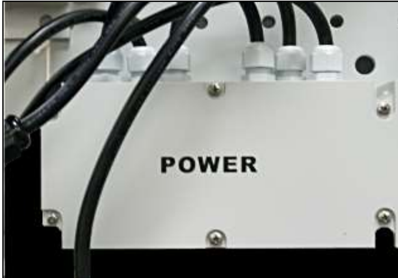
Figure 4-16. Junction Box AC Power Cable Routing
