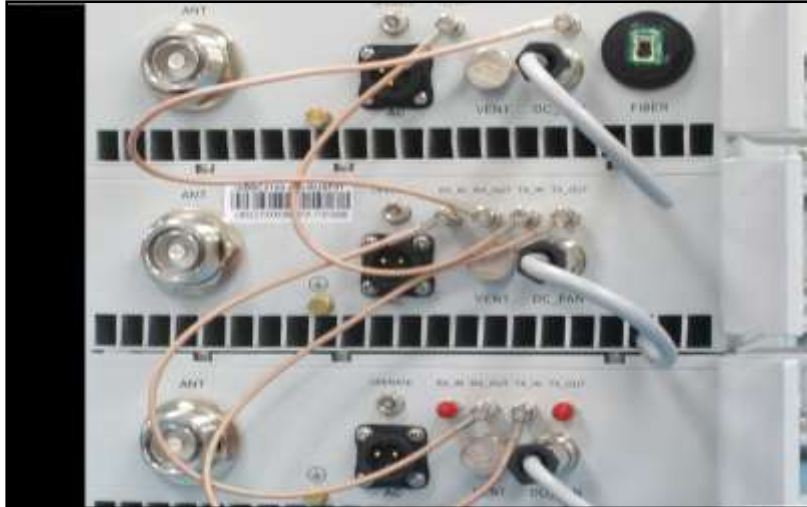
Figure 4-18. RF cable connection between Slave to Slave Remote Units
