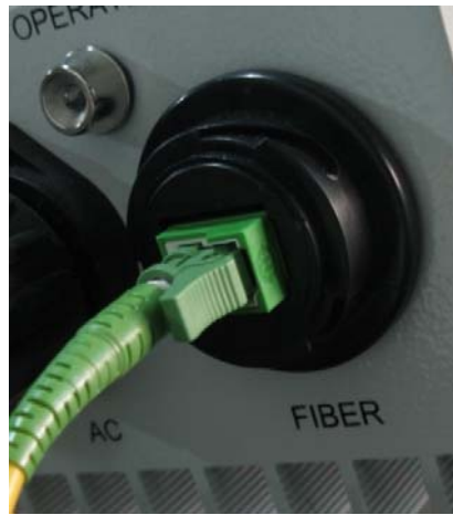
Figure 34 Fiber Optic Cable Connection to Fiber CM-BTS Enclosure
