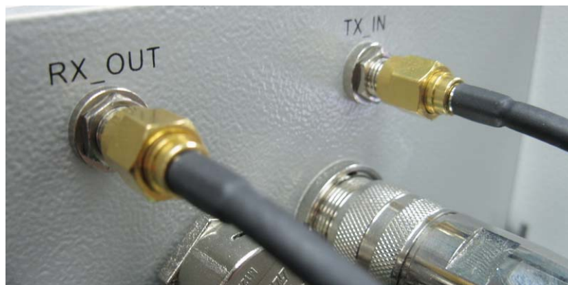
SMA Coaxial Cable Inter-connection on Single-band Enclosure
