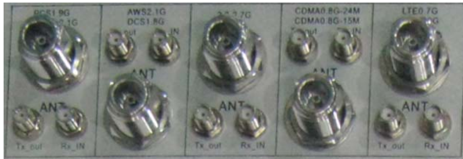
SMA Coaxial Cable Inter-connection on Fiber CM-BTS/ANT Enclosure
