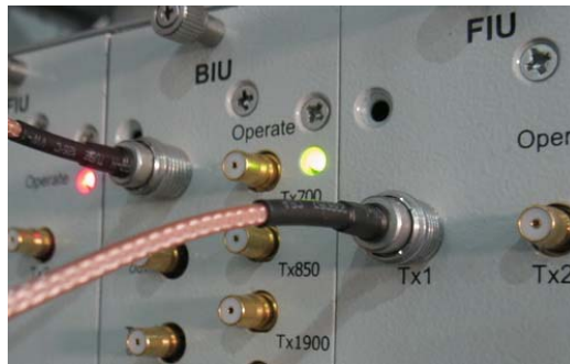
Figure 21 BTS QMA Coaxial Cable Connection
