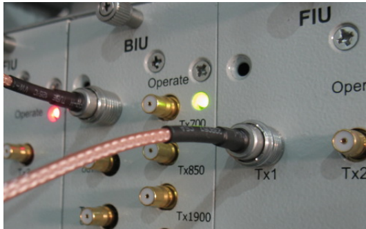
Figure 24 BTS QMA Coaxial Cable Connection
