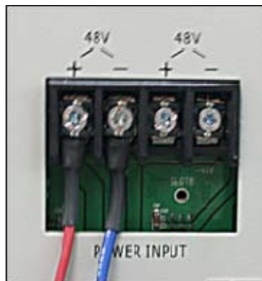
Figure 27 48VDC Host Power Connection
