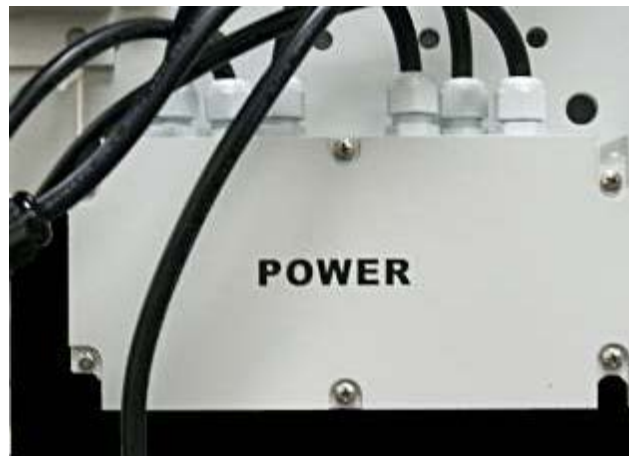
Figure 35 AC Power Junction Box
