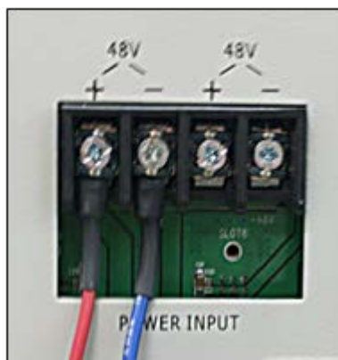
Figure 2448VDC Host Power Connection
