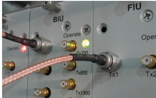
Figure 24 BTS QMA Coaxial Cable Connection
