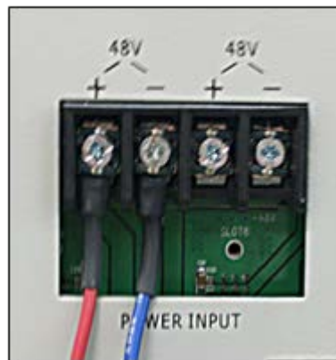
Figure 27 48VDC Host Power Connection
