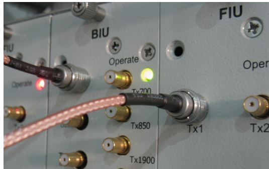
Figure 24 BTS QMA Coaxial Cable Connection
