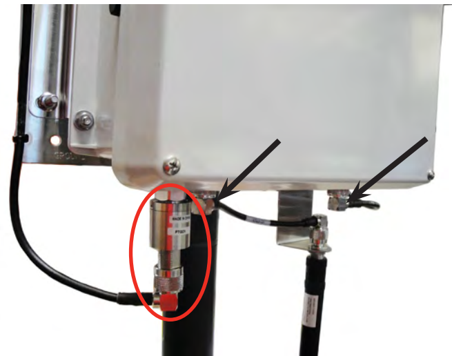
Figure 28: One attached lightning arrestor (Ground is not pictured). Arrows indicate where additional lightning arrestors should be attached.
