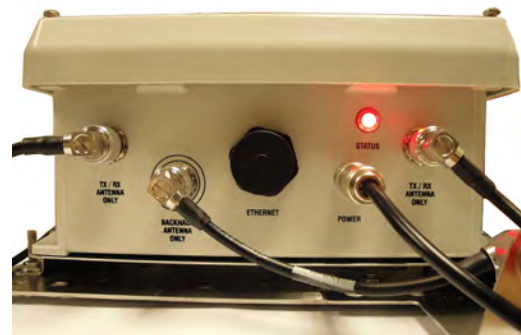
Figure 56: Gateway on battery power
