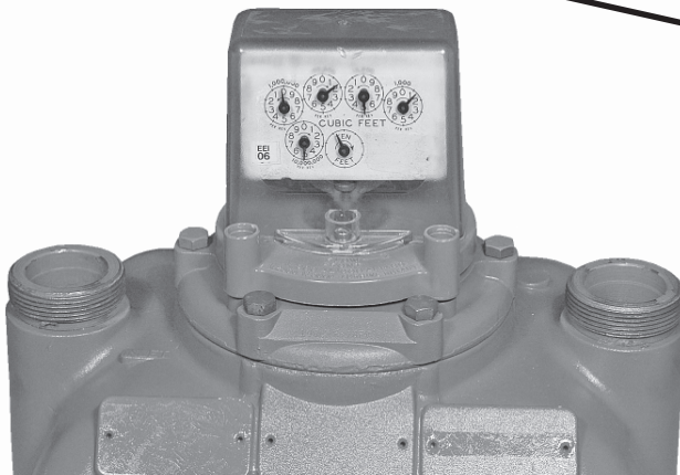
Before Installation with Red Security Seals
