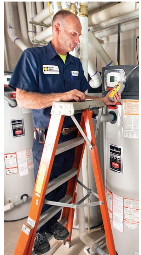
Below: A Gold Seal supervisor performs an annual maintenance check on one of many Bradford White eF water heaters at the Affinity independent living community. Dan Frisch Photography.
