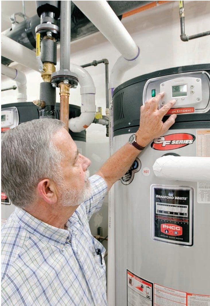
A facility manager sets the function of an eF water heater installed by Gold Seal Mechanical. Dan Frisch Photography.
