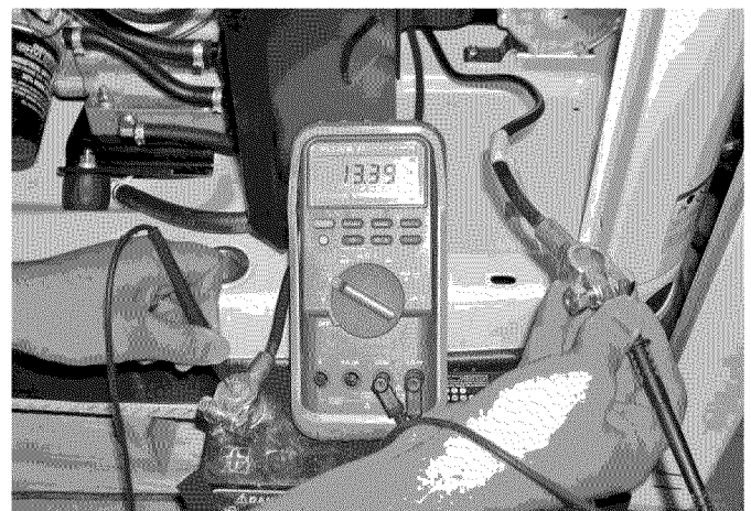
Figure 2.3 — Measurement of Charger Output with Battery Disconnected
