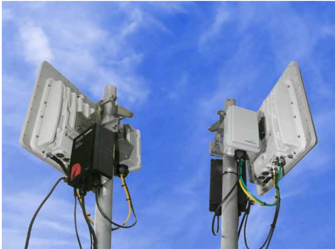
Figure 130- GPS Synchronization Unit Complete Installation
