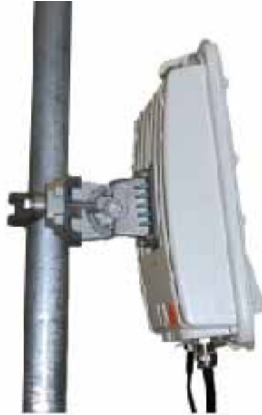
Figure 39 - ODU Mounted on Pole
