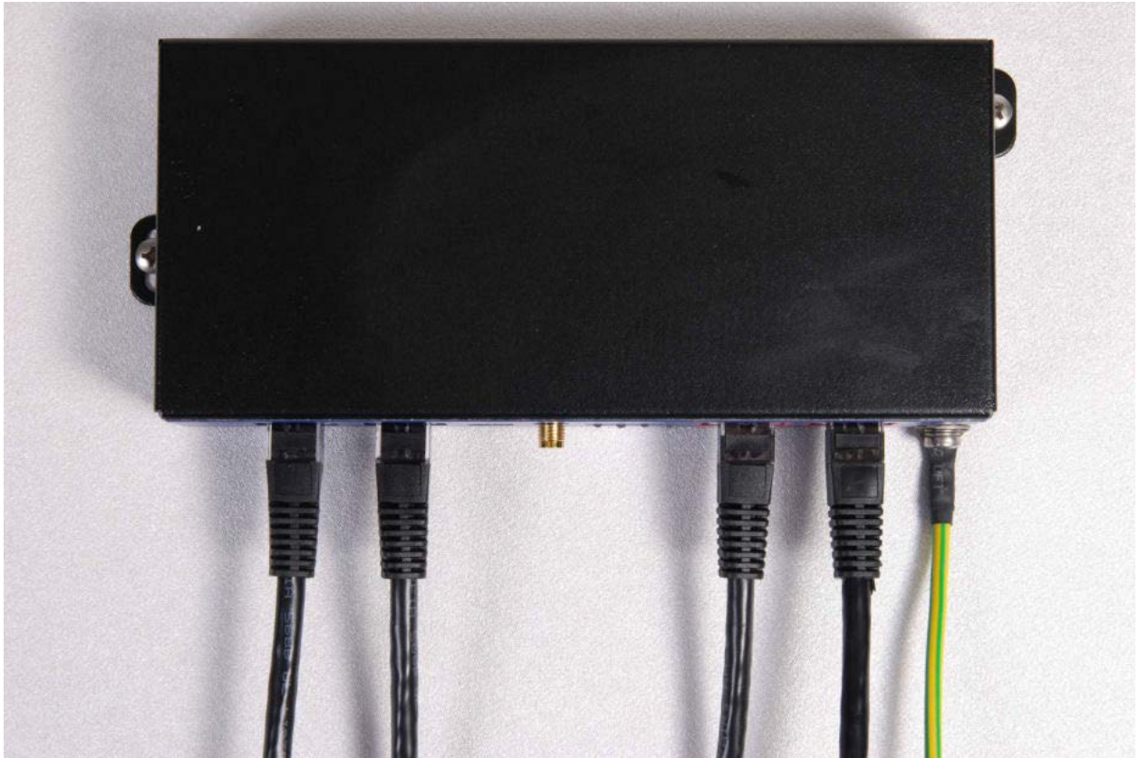
Figure 113 PTP-SYNC mounted on a wall
